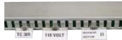
Trunking identified with PE
