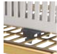
clamped to perforated plate
