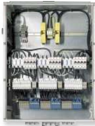
DC combiner box
